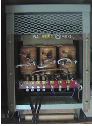
Fig. 7. Three phase transformer used in these experiments.
