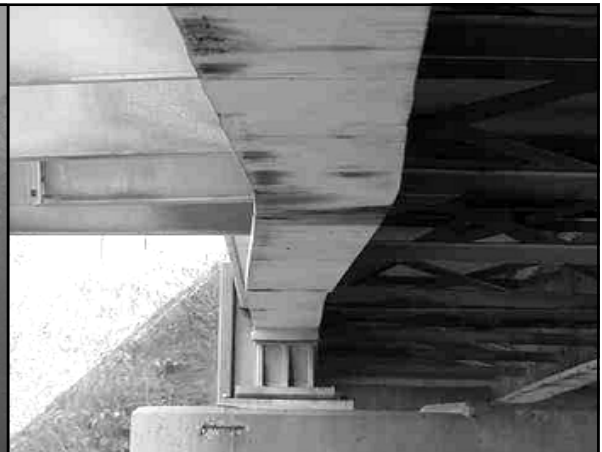
This bridge on Michigan 127 shows a damaged girder that was later repaired by heat-straightening.
