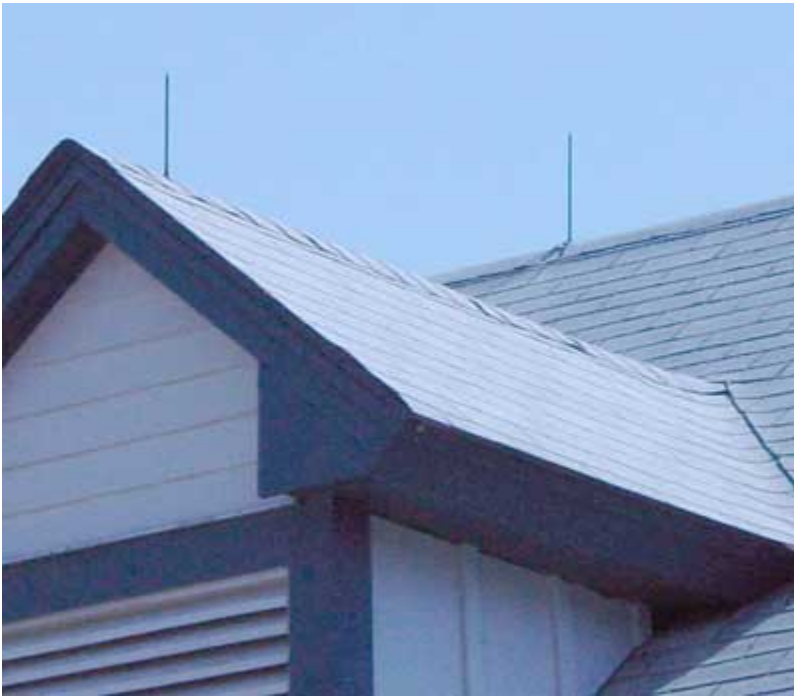
Figure 1. Attach air terminals (lightning rods) to the roof ridge to intercept a lightning strike to the building.
