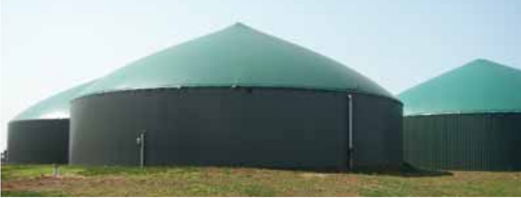
Scenic View Dairy Digester, Fennville, Mich.
