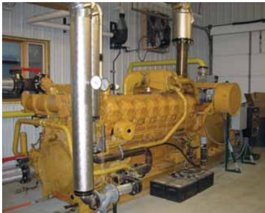
An 800 kW generator at Green Meadows Farms, Inc., ready to produce electricity, runs on biogas produced by the ADs.
